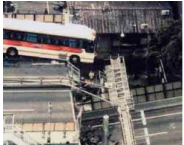
Fig. 12: Deck slab of elevated road displaced due to support movement during the Hyogo Ken Nambu earthquake of 1995 leaving the bus cantilevering precariously
