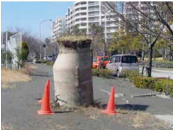
Fig. 10: Manhole above ground during East Japan earthquake of 2011 at Tokyo 373 km away from epicentre. (Photo: Prof. Towhata)
