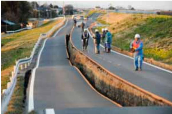
Fig. 9: Half of the highway on gentle slope experienced slide while the other half was intact during the East Japan earthquake of 2011
