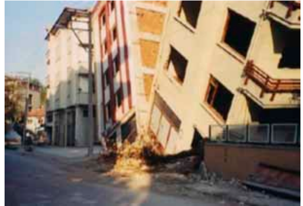
Fig. 11: Two apartment buildings leaning in opposite directions because of ground liquefaction during Izmit earthquake of 1999
